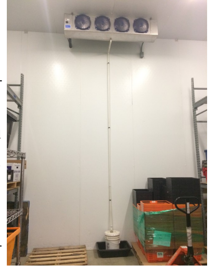
This cooler has no floor drains. Instead the evaporator drain is plumbed to a bucket that is emptied according to an SOP.
